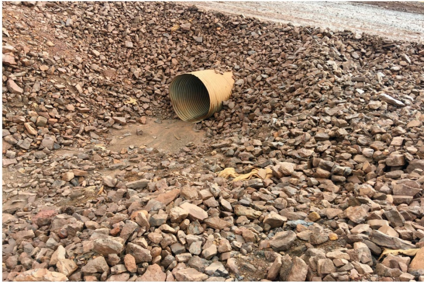
Photo 9 : Culvert under site access road (Mine / contact water ditch) - Metal sheet partly obstructing culvert (see detail below)
