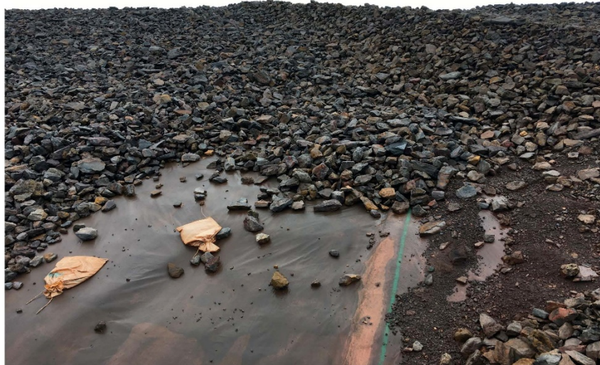
Photo 5 : Water Pond - Slumps / deformation in upstream side of south dyke (i.e. inside the pond) exposing bituminous membrane in 5 locations
