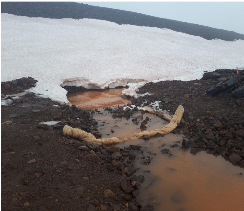
Exfiltration from repair section passing through filtration sock
