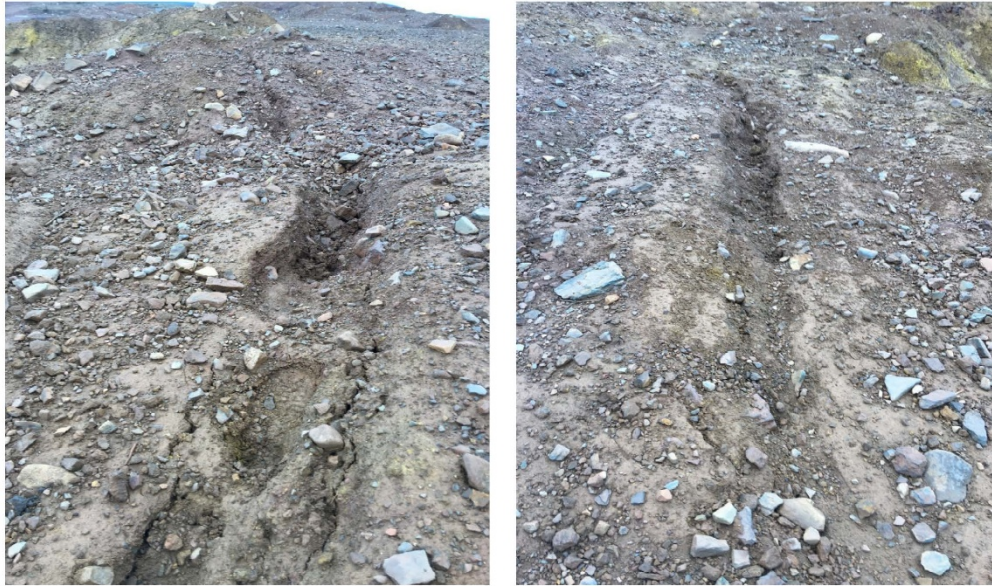
Photo 3 : Waste Rock Dump (inactive < 2020 portion) Settlement crack at crest of slope on northern area on a single lift. Photo looking downward.
