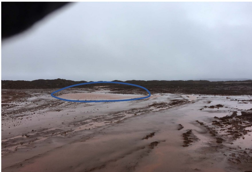
Photo 2 : Overburden stockpile (active) - Ponding on surface indicating of poor drainage
