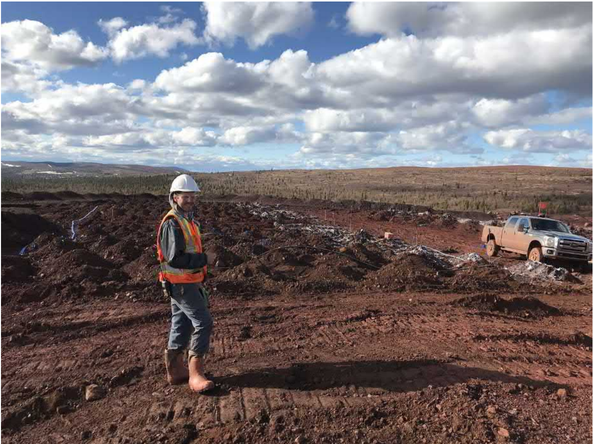
General overview of the Timmins 4 restoration block 2 (with and without rough and loose)
