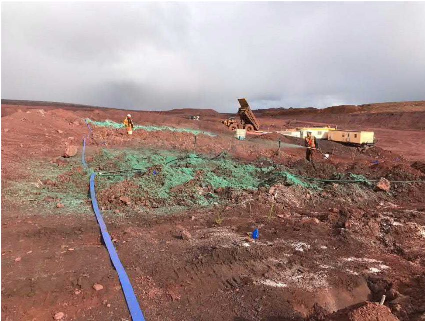
2-inch pipe (blue) primary level and restoration block 1 irrigation system overview
