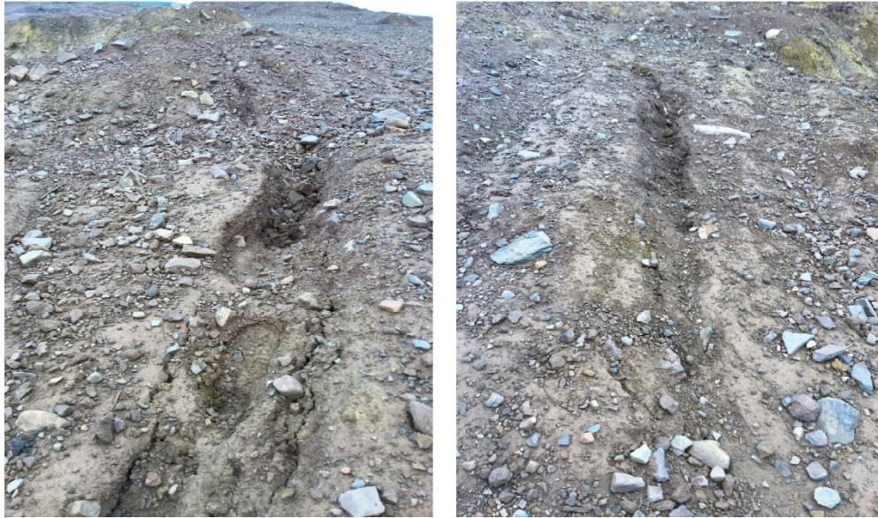
Photo 3 : Waste Rock Dump (inactive < 2020 portion) Settlement crack at crest of slope on northern area on a single lift. Photo looking downward.
