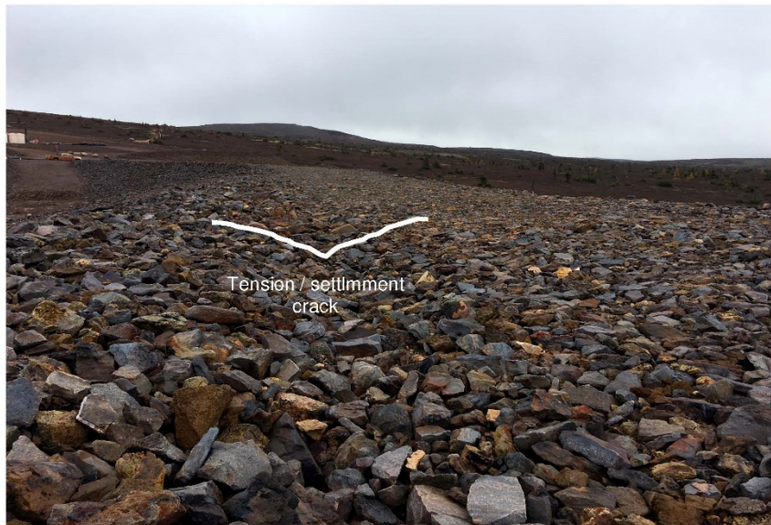
Photo 6 : Water Pond - Tension / settlement crack on south dyke as observed summer 2019
