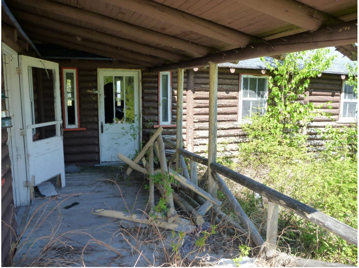
Photo 14: Abandoned building at Vieux Poste (2012, Nathalie Girard, MFFP).
