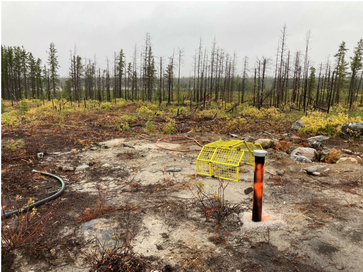
Figure 8 Typical monitoring well installation with protective HDPE casing on surface
