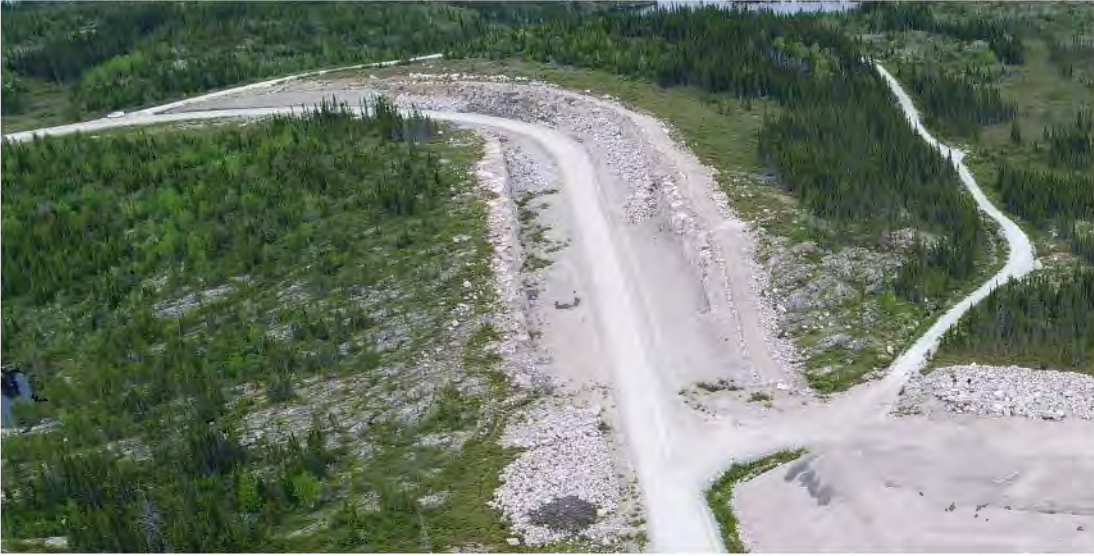
Figure 15 - Aerial view of the R6 winter road section on the right, from the permanent road to the center with on either side, the C-07 quarry, in 2017
