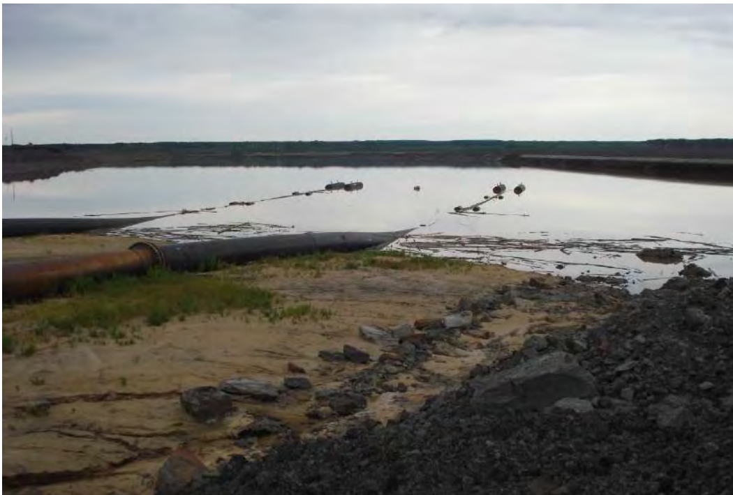
Photo 2.2: Siphon Intake Floating in Pond
