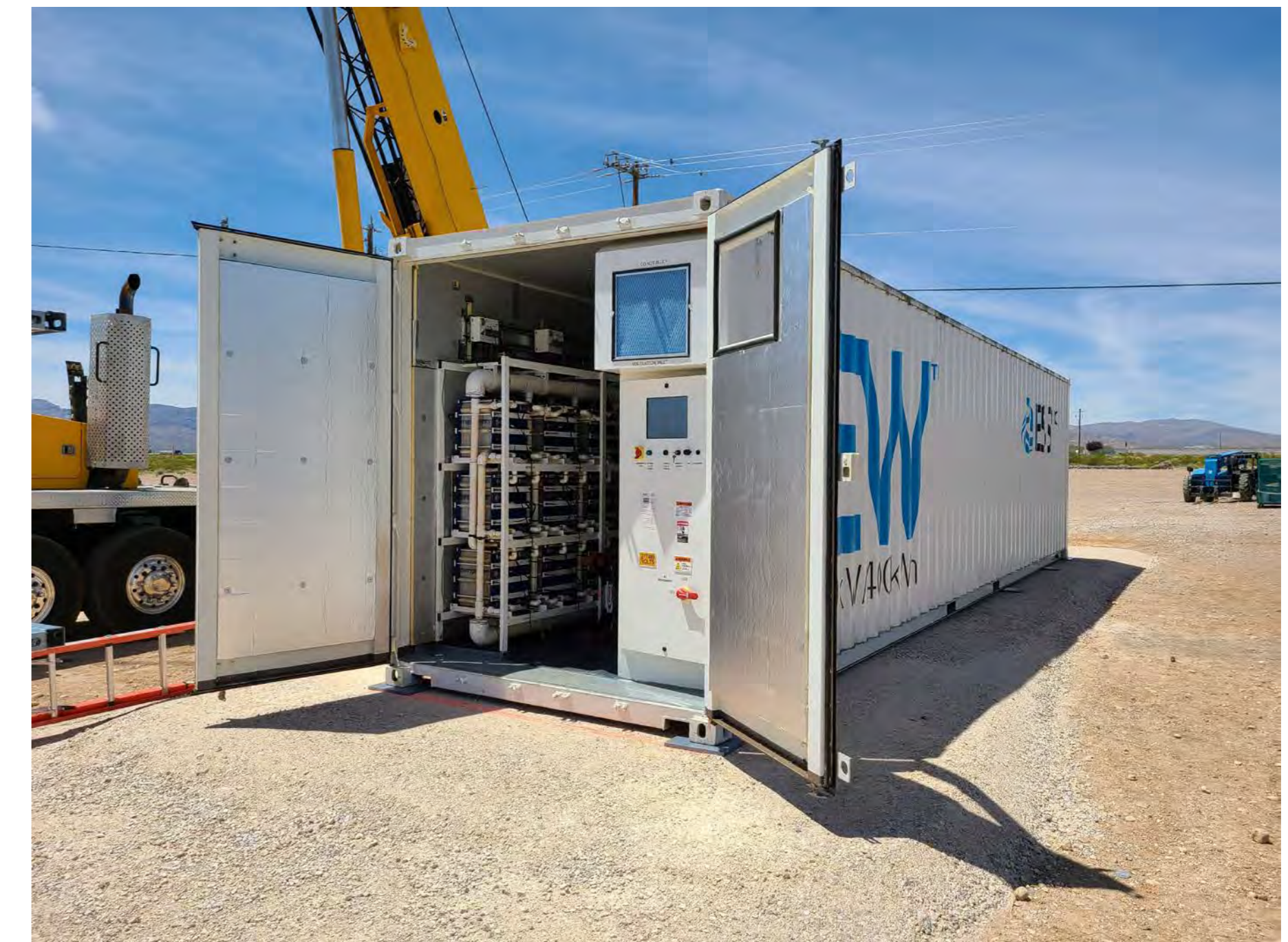
Exemple d'installation de batteries de stockage / Example of a storage battery installation, © Photo ESS Tech
